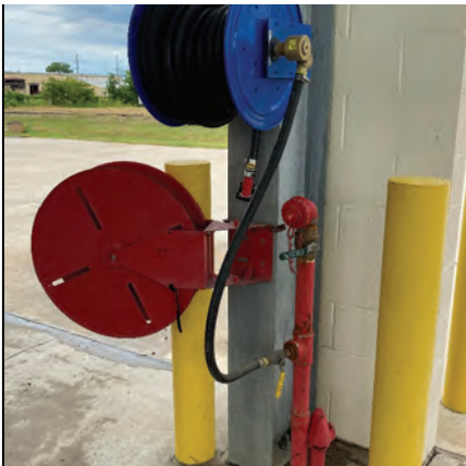
4 interior hydrant locations with 3/4" water hose connection, equipped with manual hand crank hose reel for storage, and 2.5" NST connection for fire hose.
