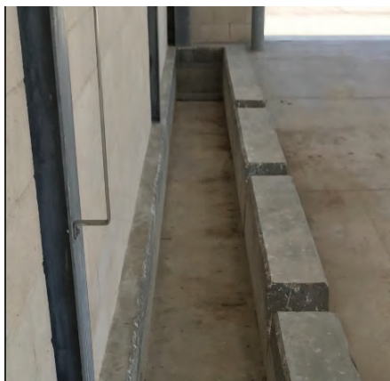
Building drainage leading to Sand / Mud Interceptor, which intercepts the wastewater and retain it for a sufficient amount of time.
