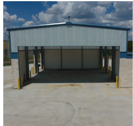
Different equipment and features are continually being evaluated and installed for ease of operation and safety.
